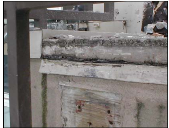
Balcony Damage Where Flashing and Railings Were Removed After Inspection
