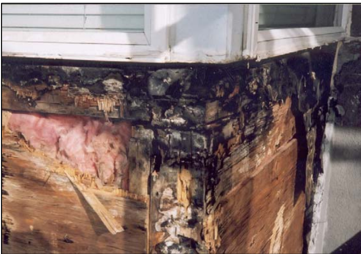
Wood Rot Discovered Behind Siding beneath Windows
